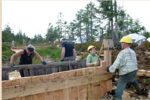
The volunteers performed impressive work during the two restoration weeks – as seen here as they construct a new pile wall.
