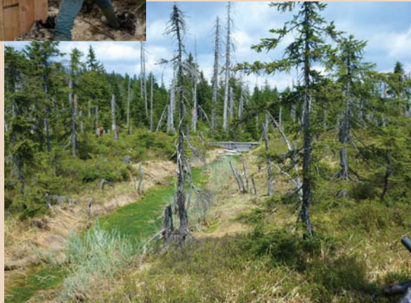
Before: The over 20-year-old pile walls were now only partially effective.
